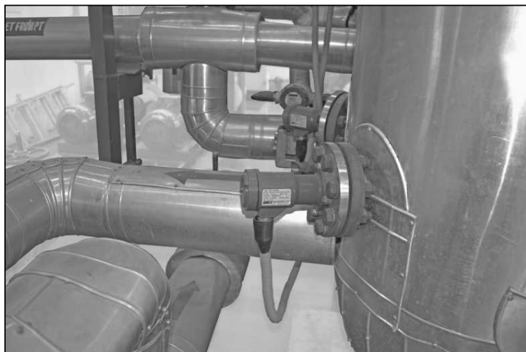
Figure 4.37 Level switch installed in the bottom of the tank
