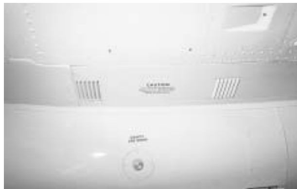
8. INVERTER COOLING LOUVERS—CHECK
