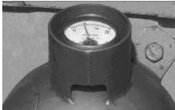
7. FIRE EXTINGUISHER PRESSURE (IF INSTALLED)—CHECK
