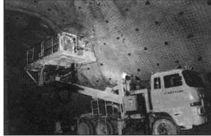
Figure 3.4. Underground petroleum storage facilities.
