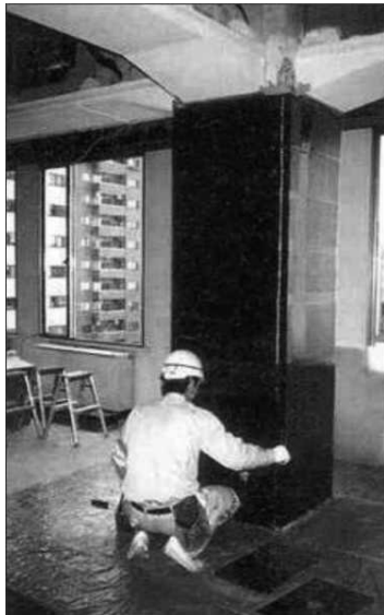
Figure 3.6. Fiber sheet jacketing of building column.
